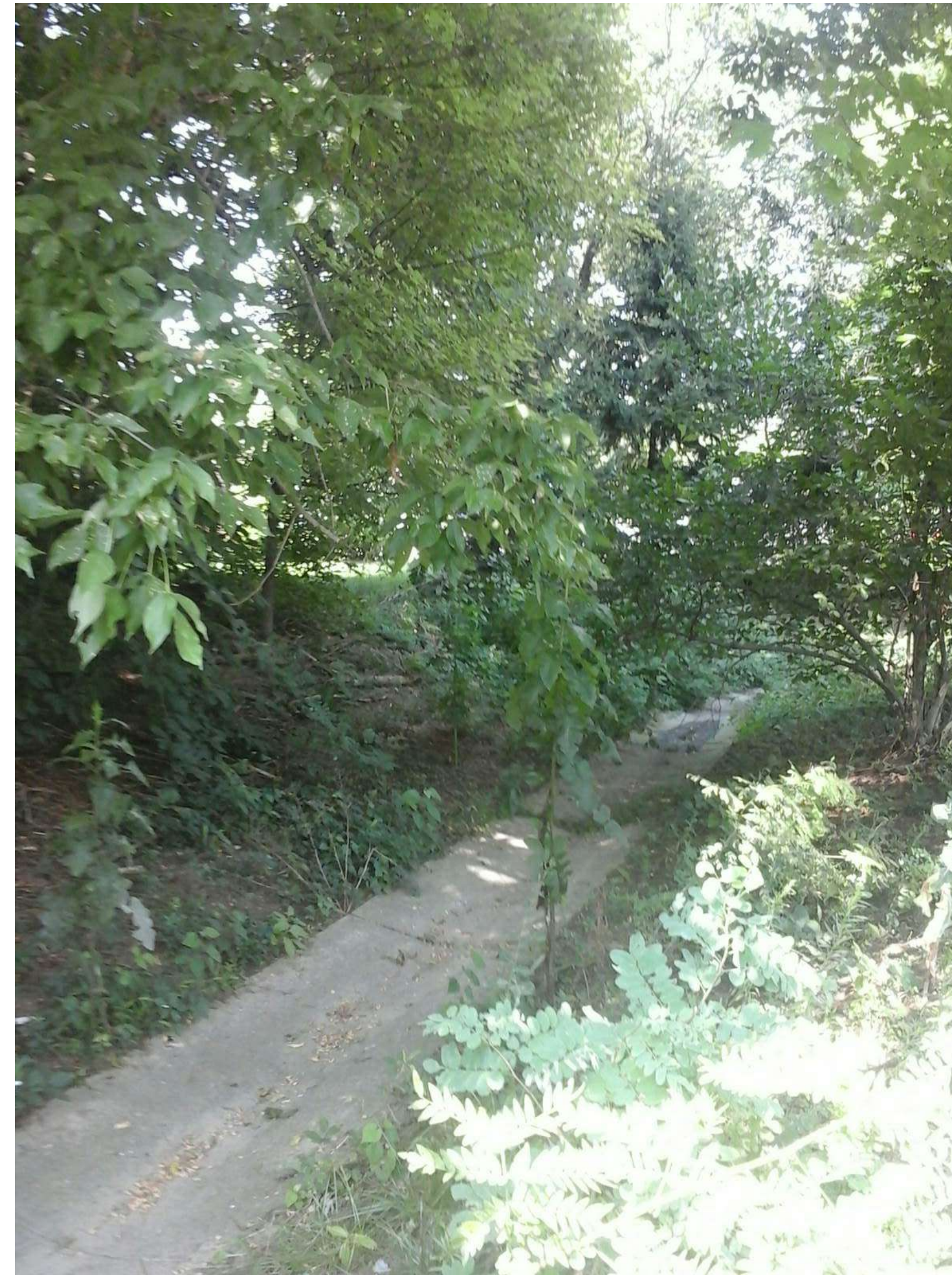
Sediment in low flow channel
