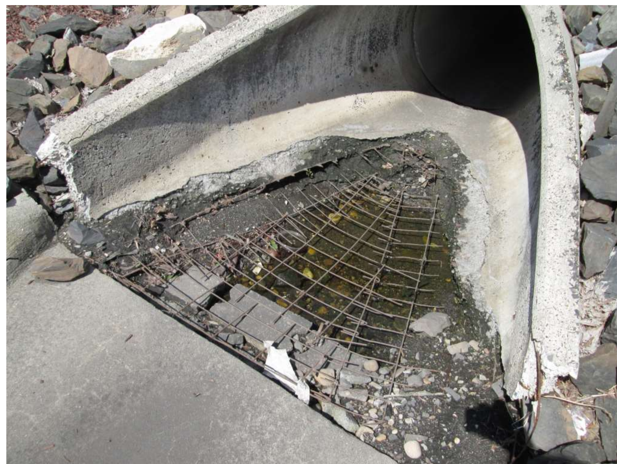
Erosion of inlet
