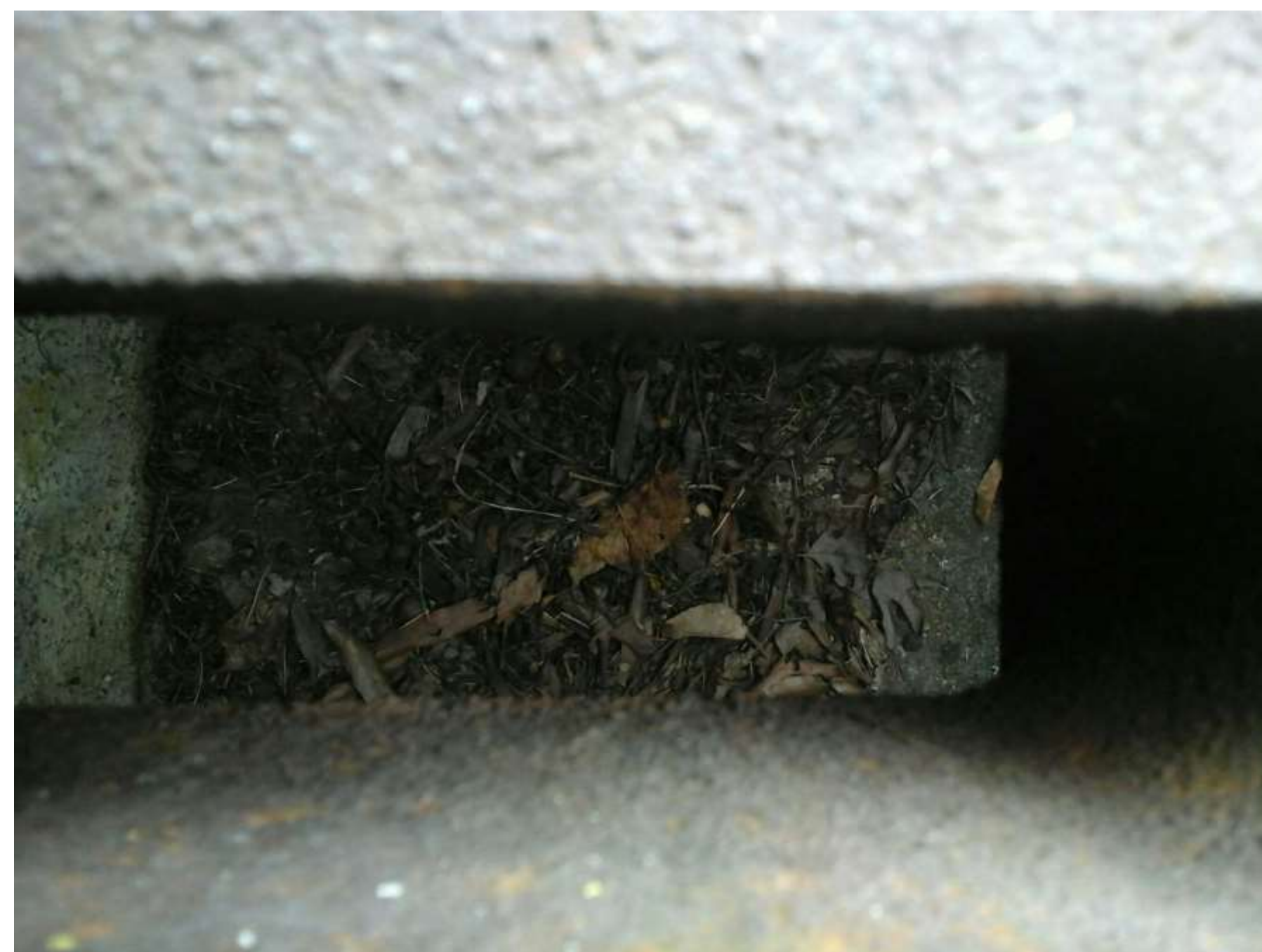
Sediment in outlet
