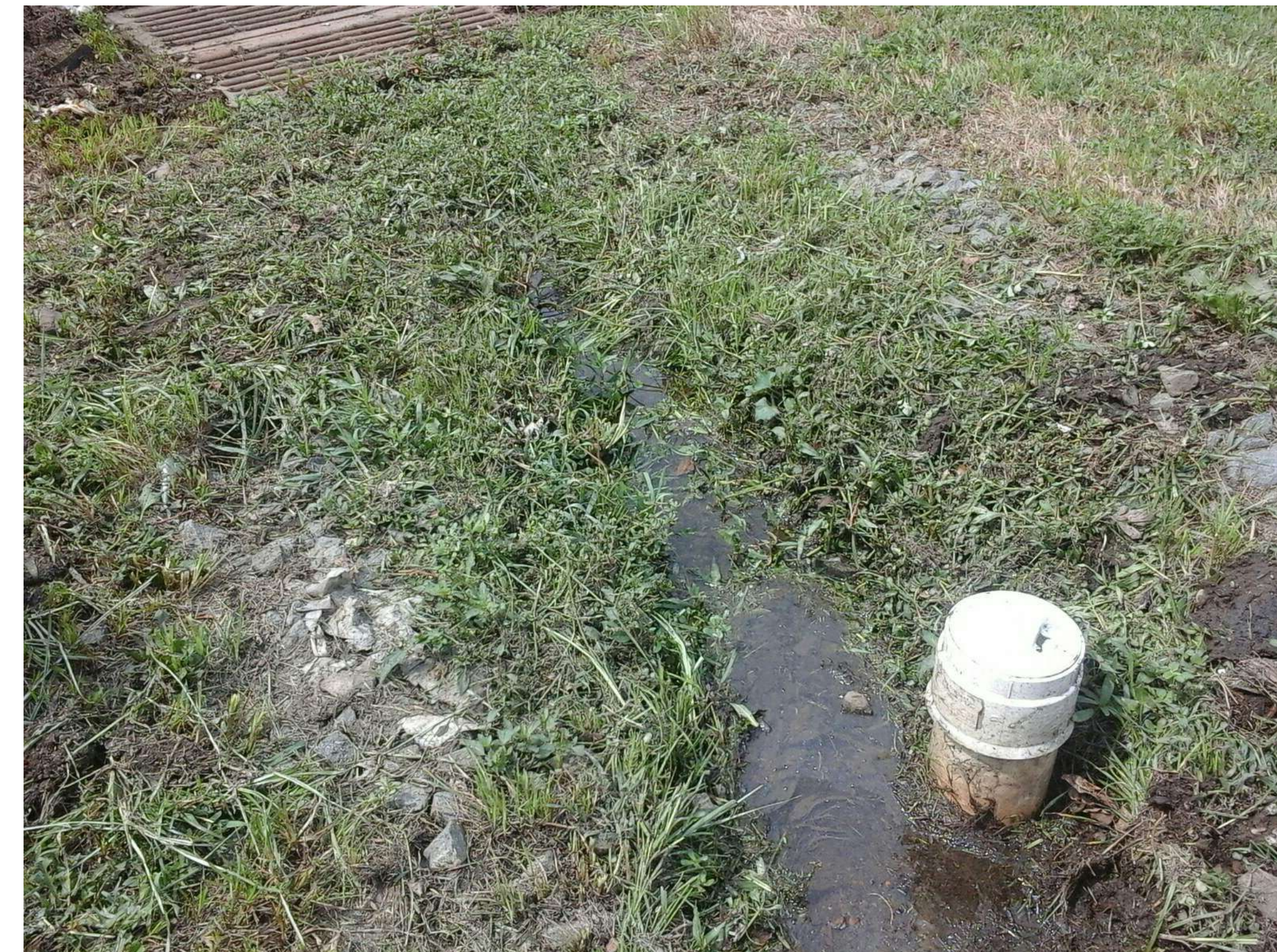
Clean out in low flow channel
