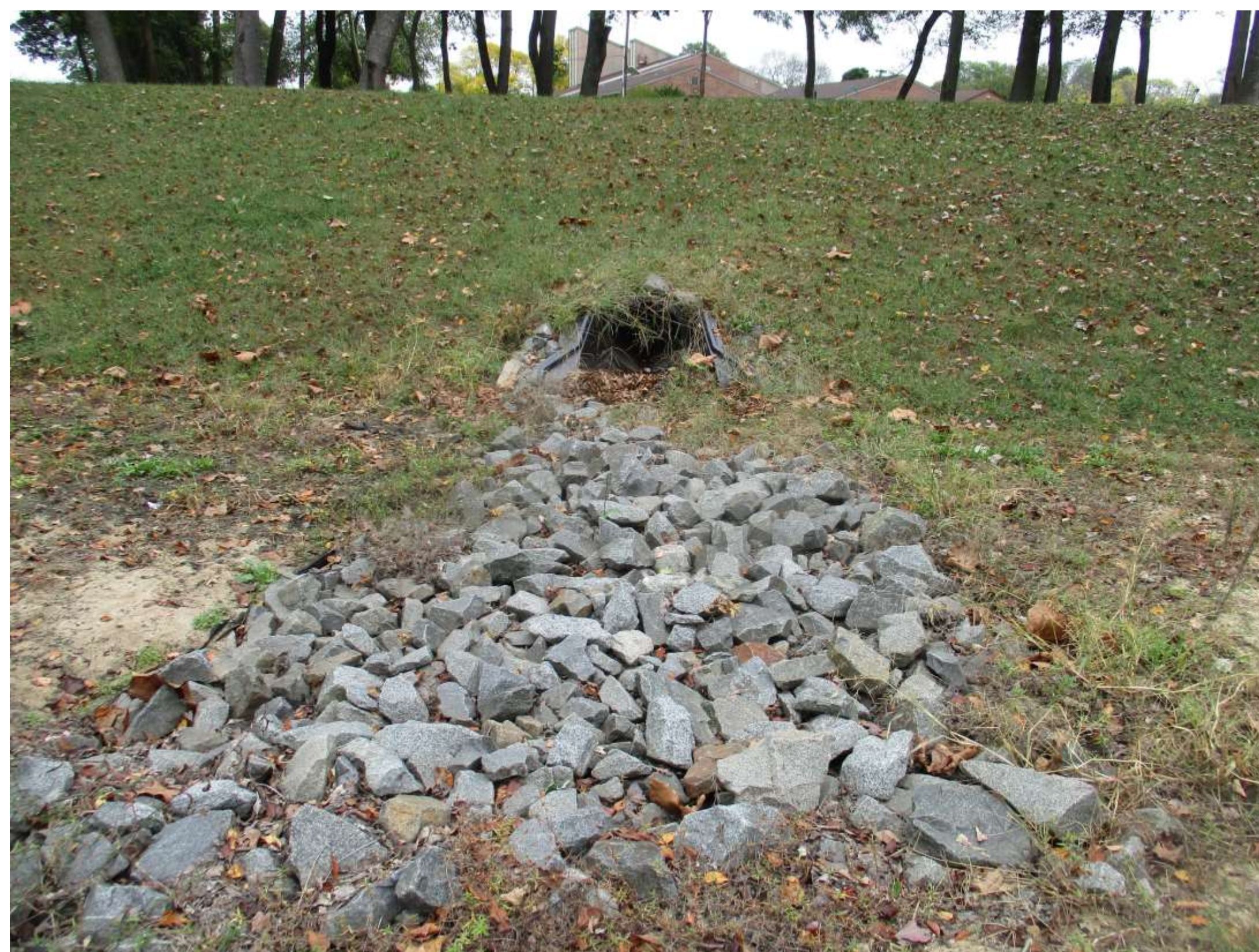
Inlet with rip rap
