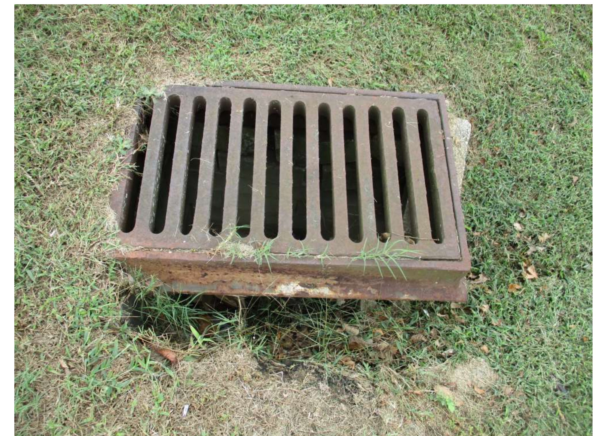
Outlet of 372 (southern basin) broken
