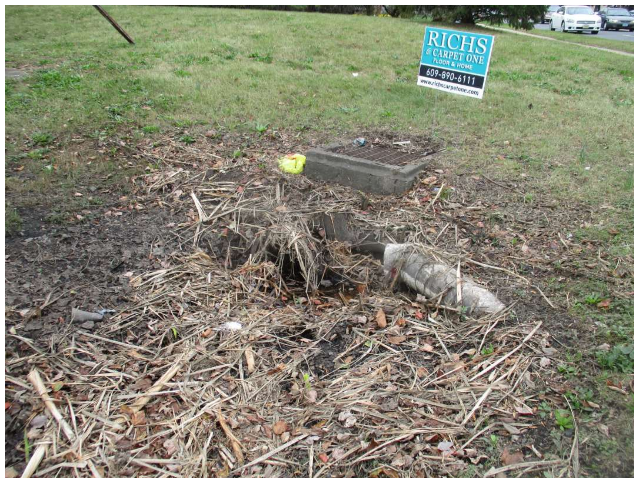
Sediment in outlet
